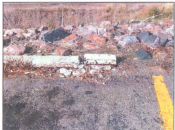
Crumbled and/or broken parking blocks are also somewhat frequent.
