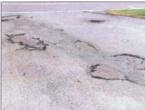
On-site street surfaces in need of repair are the most common site problems in the Survey Area.
